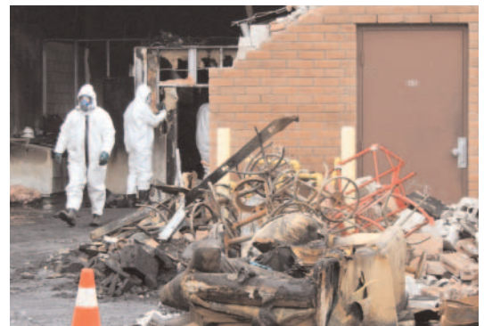
In November 2006, an explosion and fire destroyed an industrial unit on Clements Road in Pickering. The remains of a clandestine methamphetamine "super lab" were discovered with dozens of drums of precursor material and 137 kg of finished product. The finished product alone had a street value of $1.37 million. The toxic mess resulted in the permanent closure of several adjoining businesses as specially-equipped hazardous material teams had to go in and clean up the mess.
